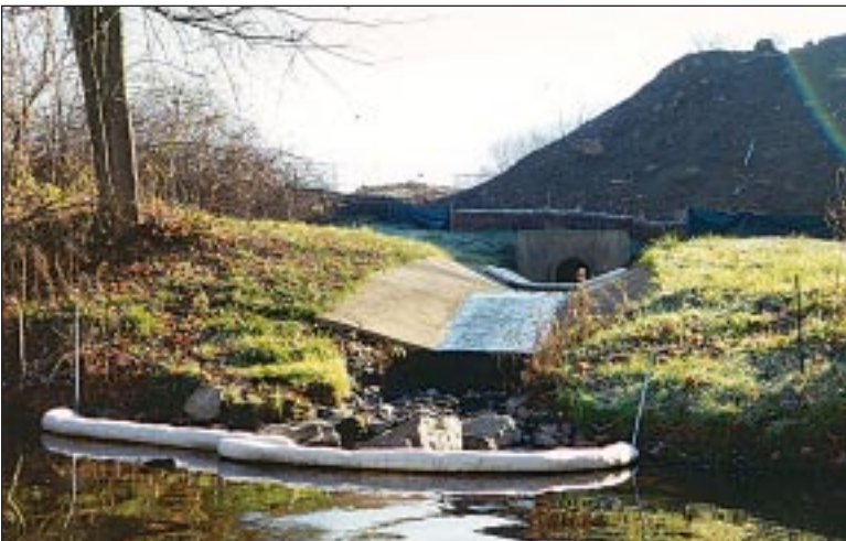
Stormwater outfall to the river
